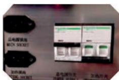
seperate machine heating power supply
